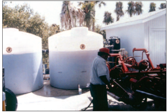
Figure 8: Recycling washdown system.
